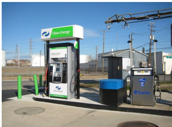
CNG station installed at an existing gas station in Richmond, Virginia. Photo from Margaret Smith, DOE, NREL 28005
