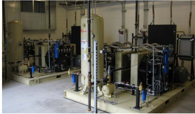
Redundant compressors at Washington Gas in Springfield, Virginia. Photo from Margaret Smith, DOE, NREL 28171
