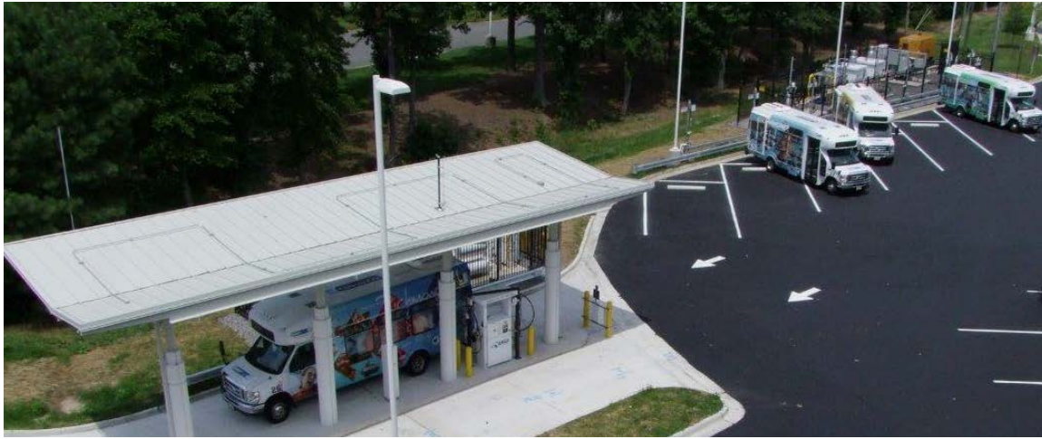
This combination-fill station fuels 14 shuttle buses at the Richmond, Virginia, airport with 14 time-fill posts and two fast-fill hoses. The fast-fill station is in the bottom left, and some of the time-fill posts are in the upper right. Photo from Marathon Technical Services, NREL 30243
