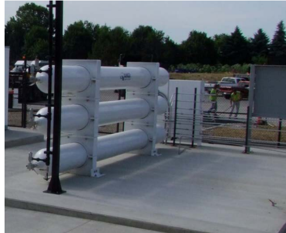
This CNG station was built with three storage vessels and has space on the concrete slab to add more storage vessels in the future. Photo from Marathon Technical Services, NREL 30345
