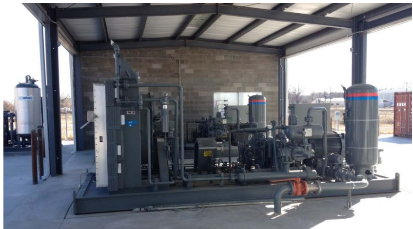
Two compressors protected from inclement weather by a canopy with easy access for maintenance. Photo from Tulsa Gas Technologies, NREL 30246
