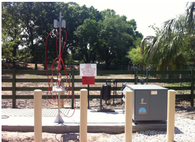
FuelMaker FMQ-8 compressor and dual hose time-fill post in Gulf Breeze, Florida. Photo from Jeremy Talbot, Phoenix Energy Corp, NREL 28228
