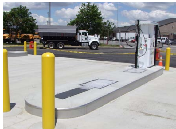
This CNG station was built with one dispenser and has concrete poured to easily install three more dispensers in the future. Photo from Marathon Technical Services, NREL 30344
