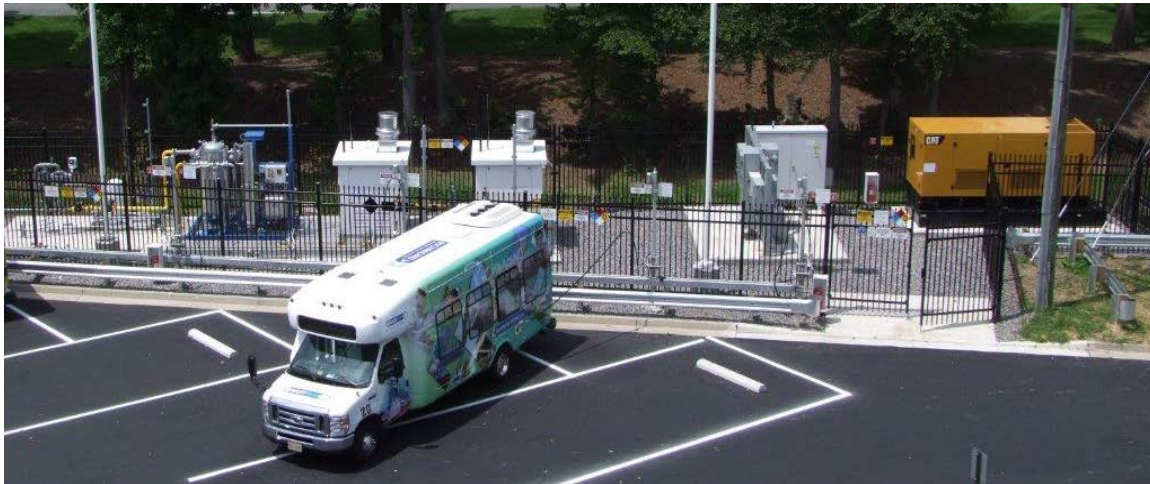
A shuttle bus fuels at a time-fill post at the Richmond Airport combination-fill CNG station. From left to right, the equipment behind the fence is a silver gas dryer, two compressors enclosed in white boxes, electrical system, and a generator at far right. Photo from Marathon Technical Services, NREL 30245
